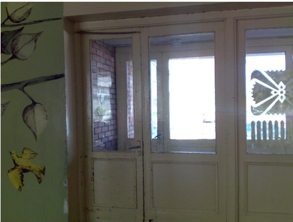
Picture 5. Low quality doors in Vyduno secondary school affects the energy performance of the building and creates cold bridges.
