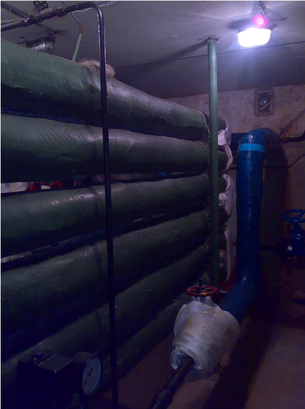
Picture 1. The old heating centre of Petrašiunai secondary school. There might be asbestos findings when renovating the old heating centres and systems.
