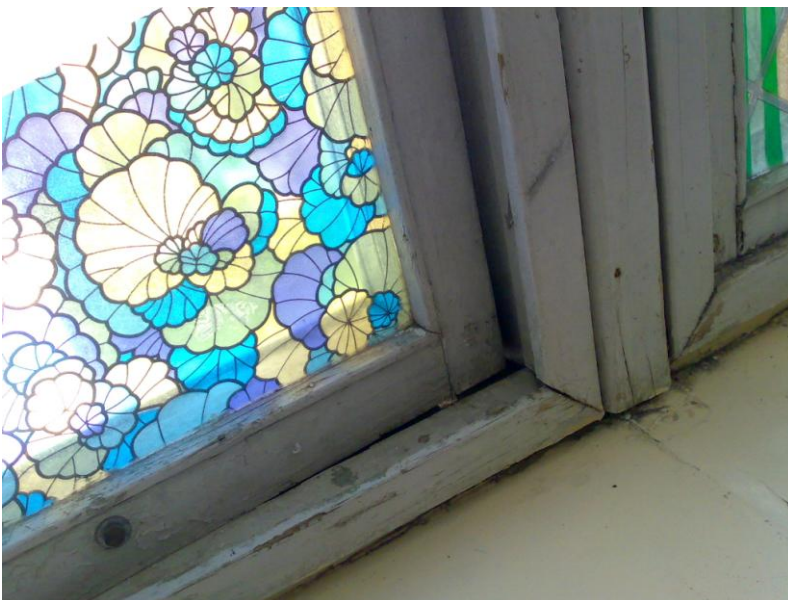
Picture 3. A window in Petrašiunai secondary school. The window does not close properly as can be seen in the picture.
