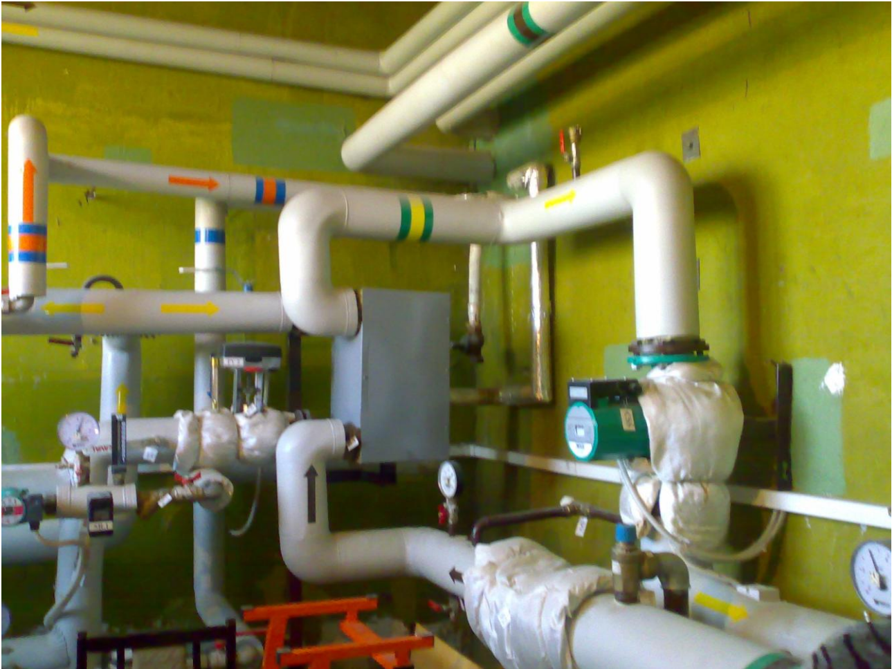
Picture 2. The renovated heating centre of Purienu secondary school
