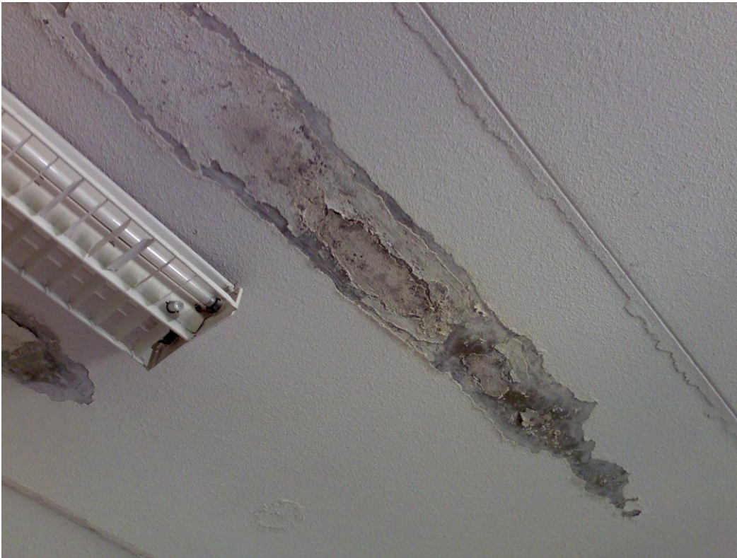
Picture 6. A major moisture damage in the roof of Petrašiunai secondary school.
